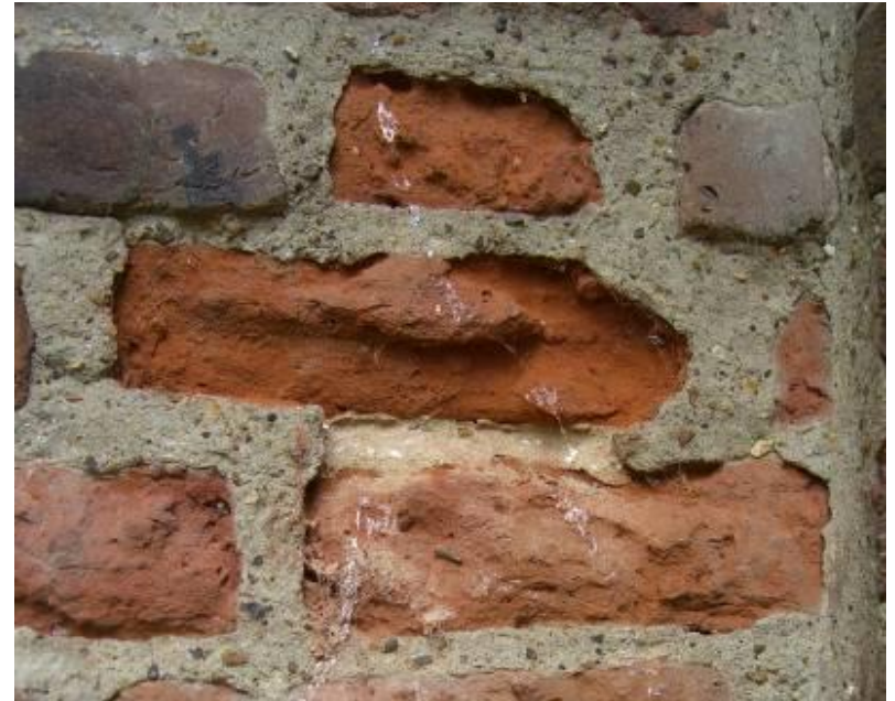
Lime mortar repointing required
