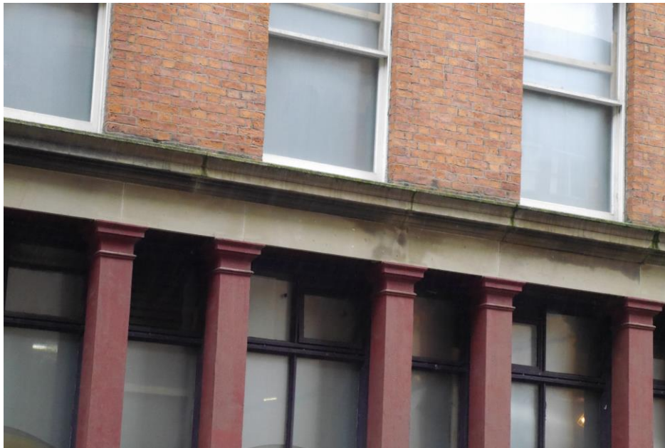
Lead capping required to ledge
